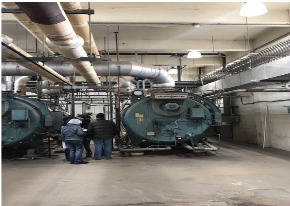
Figure 5.4. Sludge Treatment Furnace at Wichita Wastewater Facility
