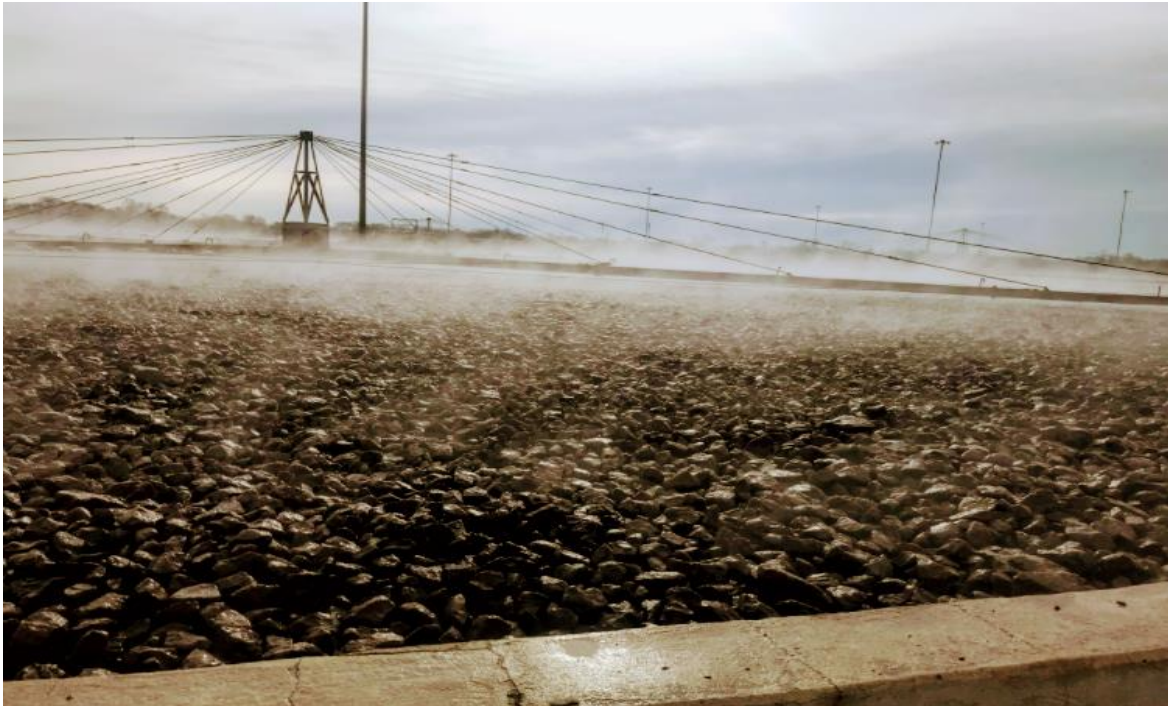
Figure 5.8. First Stage of Filtration Process (Wichita Wastewater Facility)
