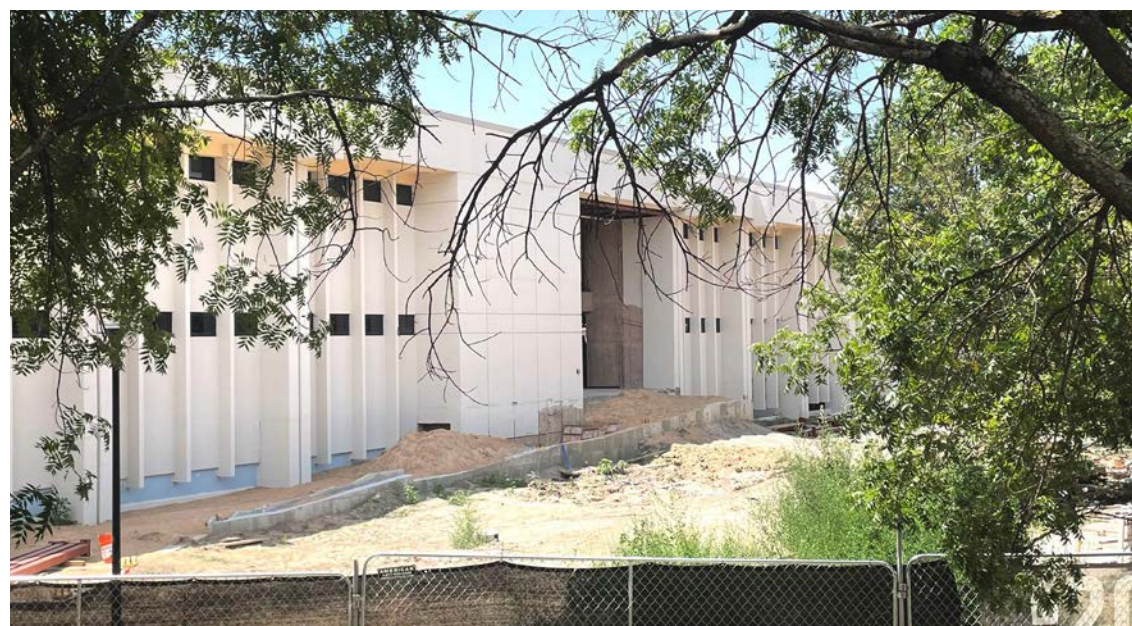
Clinton Hall construction on Aug. 3, 2023. | Photo by Nithin Reddy Nagapur / The Sunflower
