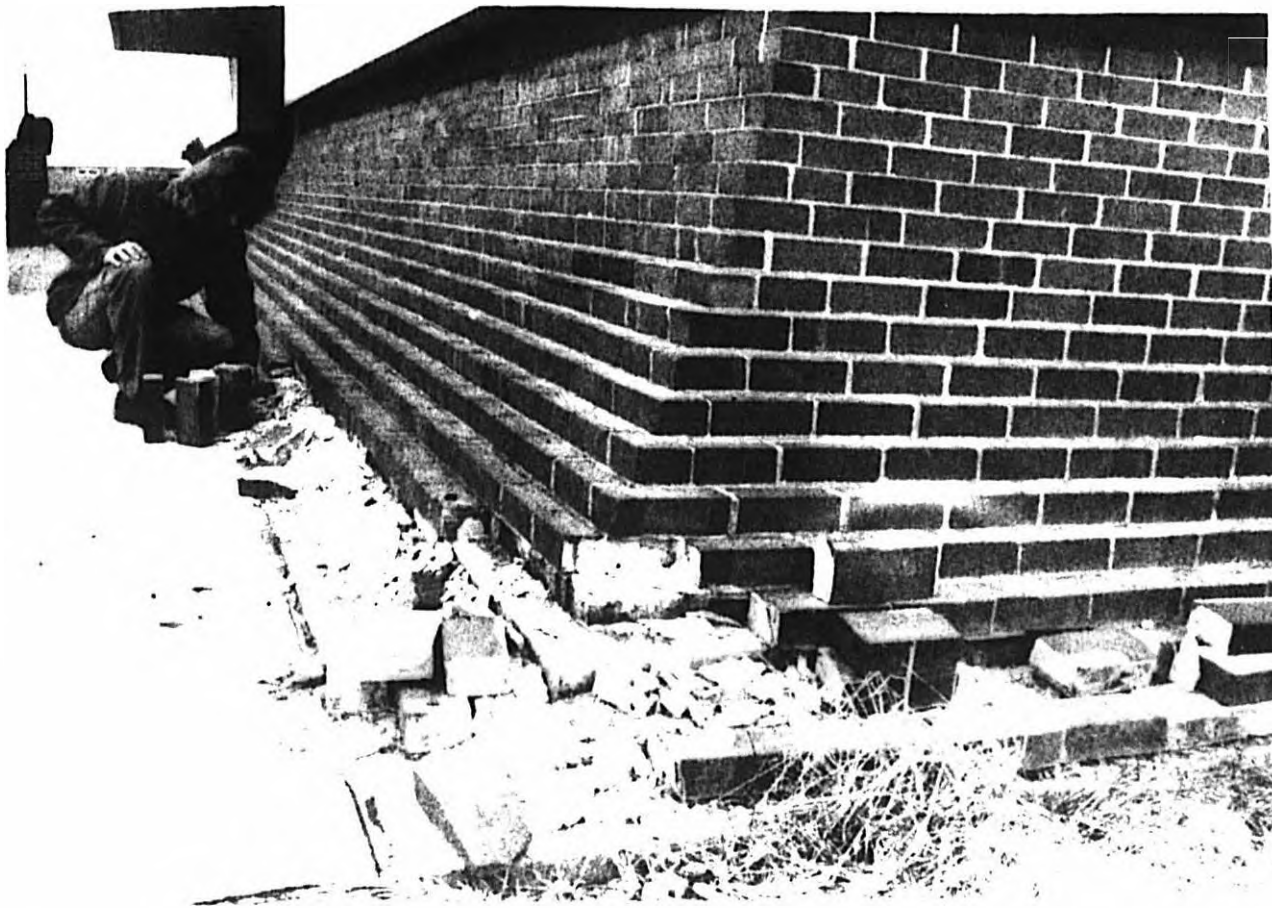
Contractors of the Life Sciences Building will not receive final payment for the construction of the building until it is considered complete. Todd Middleton looks at bricks that have already fallen away from the base of the building. (Photo by Roger Giesecke)
